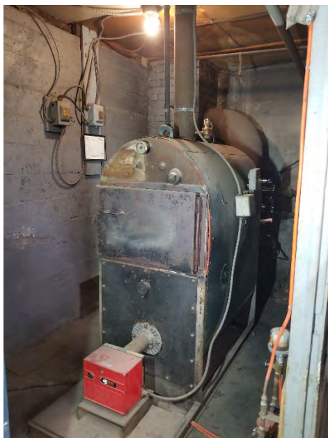
Old Oil-Fired Burner Furnace
