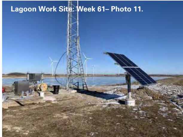
Photo 10&11: Cable connection is in progress for the Communication Antenna at the Lagoon Site.
